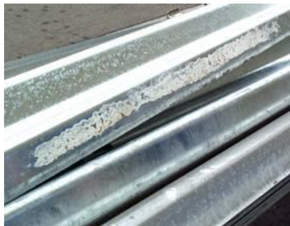
Picture 2 - White rust
