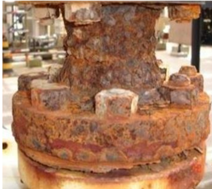
Picture 1 - Rusty flange
