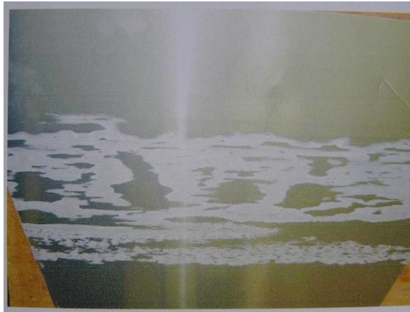
Picture 3 - White rust on aluminium
